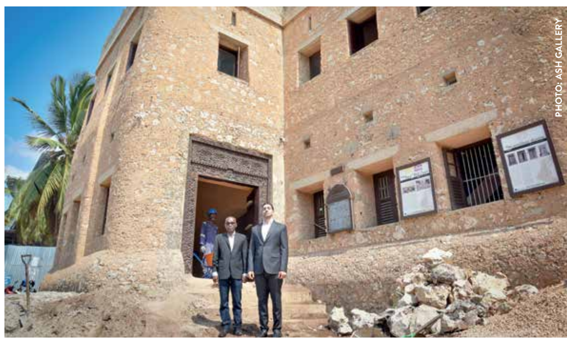
Suddenly more beautiful: chief conservator Ali Said Bakar (left) and Dubai businessmen Samuel Saba in front of cleaned walls of the historic Old Fort. The face-lift began externally. Inside, major repairs are still ongoing
